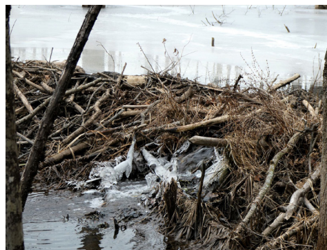
A sizable breach in the dam, photographed in January 2020, suggests that this area has been at least temporarily abandoned by beavers. The sound of running water generally triggers beavers to repair the damage.
