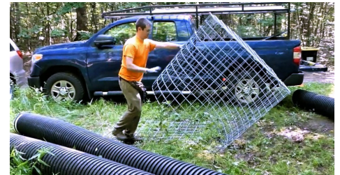
Beaver Solutions employee John Egan assembles the intake fence using heavy-gauge steel mesh.
