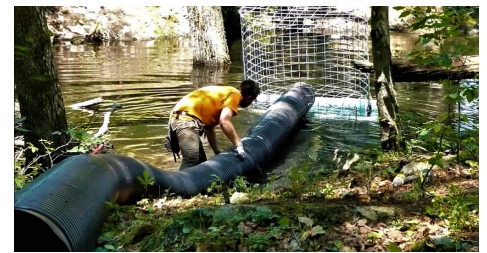
The intake fence and flexible pipe are floated into the pond on pontoons, then sunk to the bottom.
