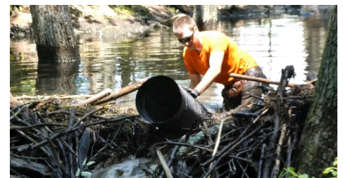
The dam is breached by hand to accommodate the pipe at the desired level, then covered over again using the same materials.
