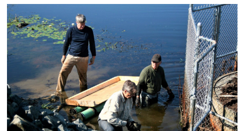
Mike Callahan led a team of BBC volunteers in 2015 to pile trap rock around the base of the chain-link fence protecting the outlet at the Fitzgerald Lake dam, to keep beavers from digging under the fence and clogging the outlet.
