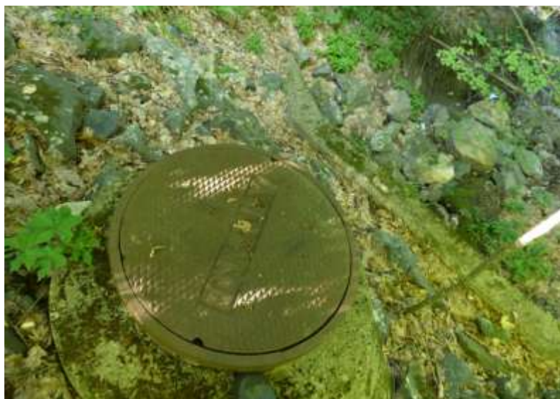
The manhole cover above the headwall for the drain from the VA.
